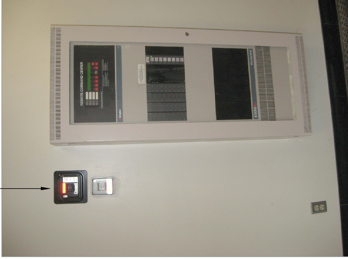
PHOTO: FIRE COMMAND CENTER
