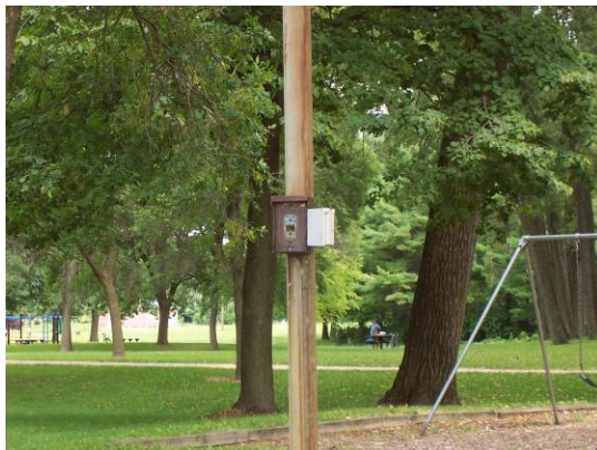
CB BOX ON POST TOP POLE
