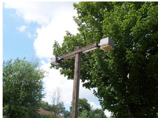
PARKING LOT LIGHTING UNIT
