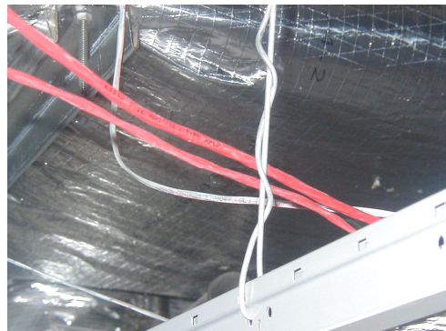
Photo #E8 – Fire Alarm Wiring
