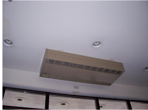
Photo #H8 – Typical electric heat in vestibule
