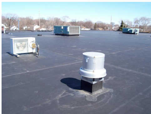
Photo #H9 – Typical roof exhaust fan
