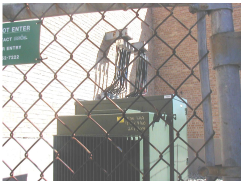
Photo #E1 – Exterior Electrical Bus Connections
