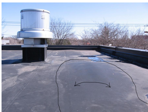
Photo #A29 – roof bulges
