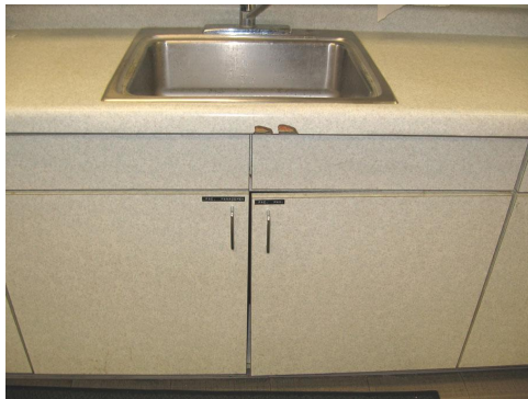
Photo #A39 – break room in Job Center
