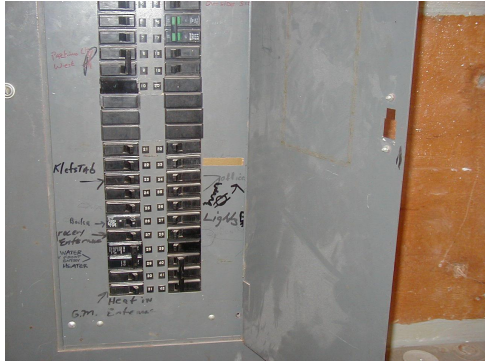
Photo #E3 – Panelboard
