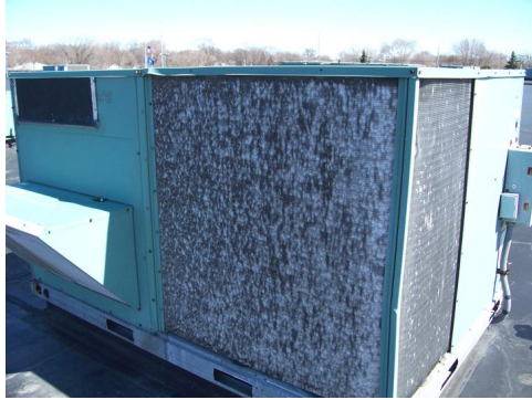
Photo #H1 – Typical hail damage to RTU coil fins
