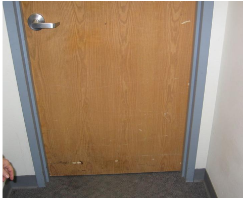
Photo #A31 – heavy traffic corridor doors
