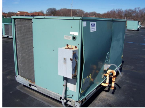
Photo #H2 – Typical RTU damage
