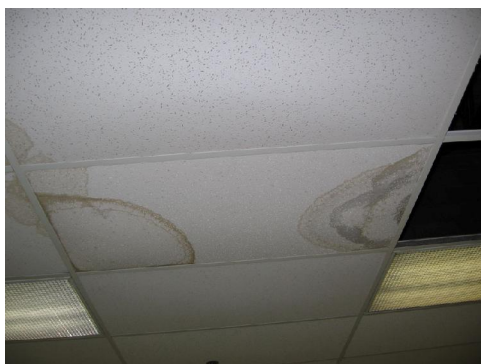
Photo #A35 –interior ceiling tiles in school
