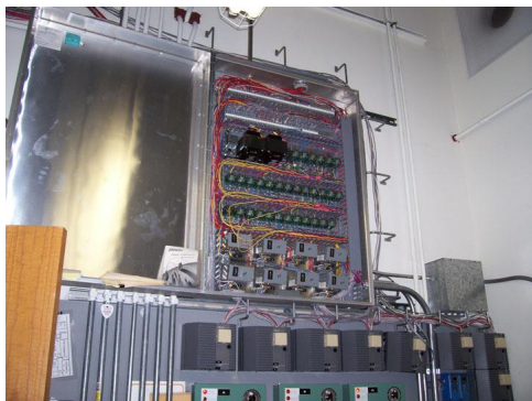
Photo #H11 – Building control system
