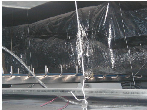
Photo #E5 - Cable Tray
