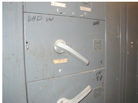
Photo #E2 – Main Switchboard Bad Switch
