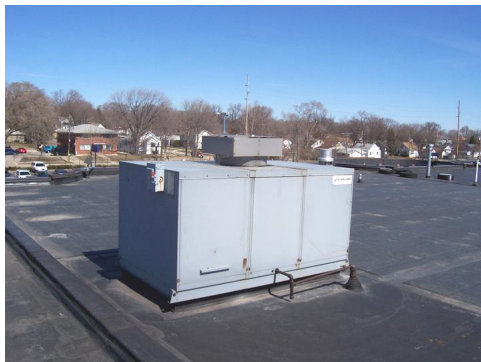
Photo #H3 – Typical heating only RTU
