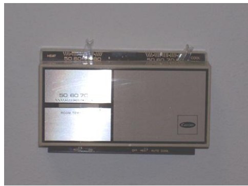
Photo #H10 – Typical non-programmable thermostat
