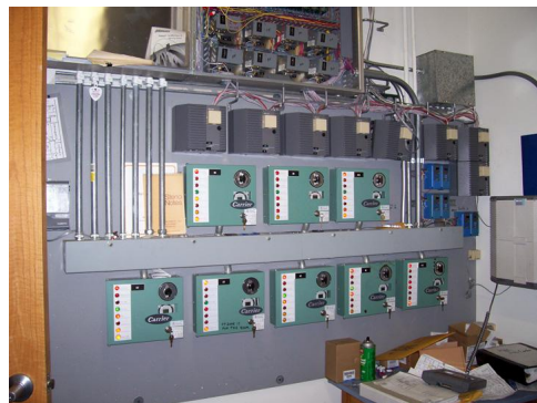
Photo #H12 – Building control system
