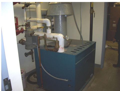
Photo #H5 – Pre-heat coil boiler
