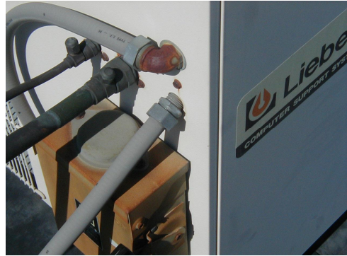
Photo #E4 – Electrical Fitting
