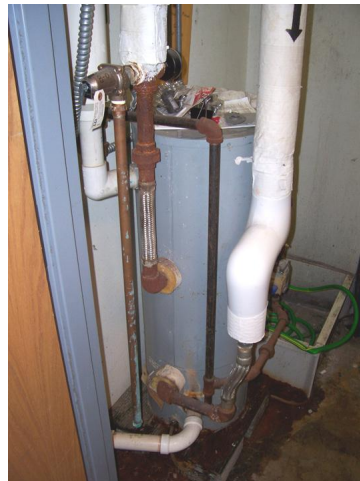
Photo #H4 – Boiler near front entrance
