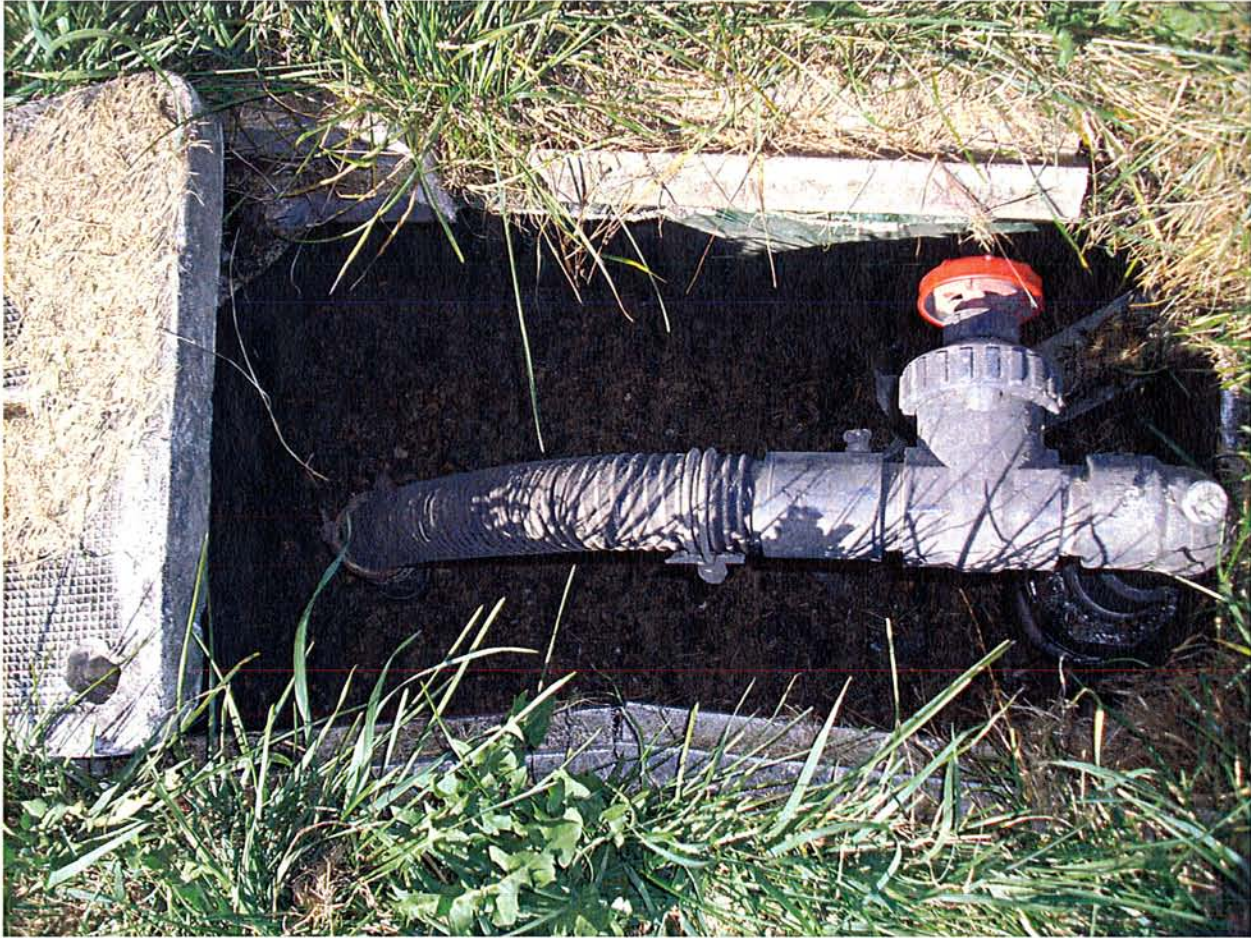
View of damaged vault box due to settlement and/or traffic.
