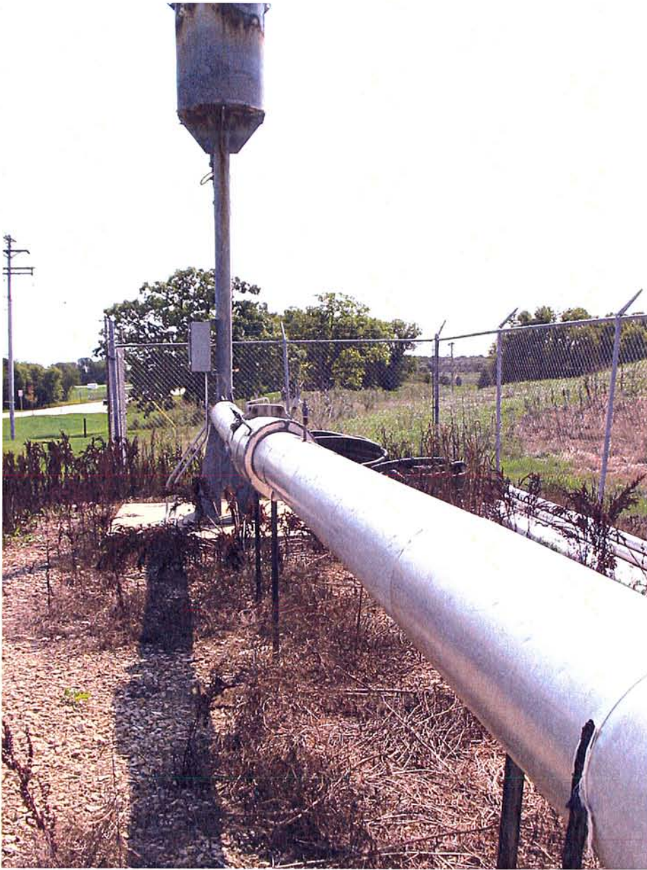
View of utility flare at Truax Landfill. Shroud is cylindrical top to flare that is secured by several bolts. Shroud has pick-holes for lifting off of flare top.
