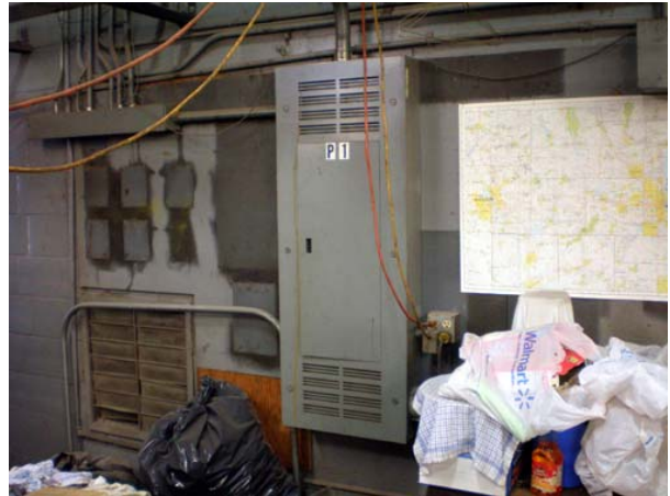
Figure 2 Electrical Subpanels (inside)
