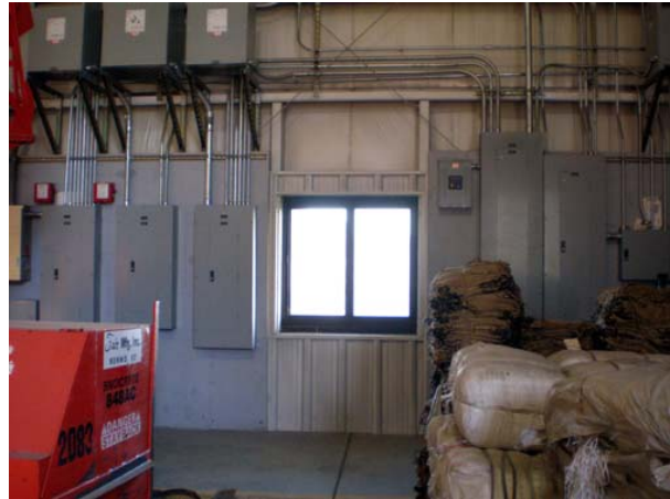
Figure 2 Electrical Subpanels (inside)
