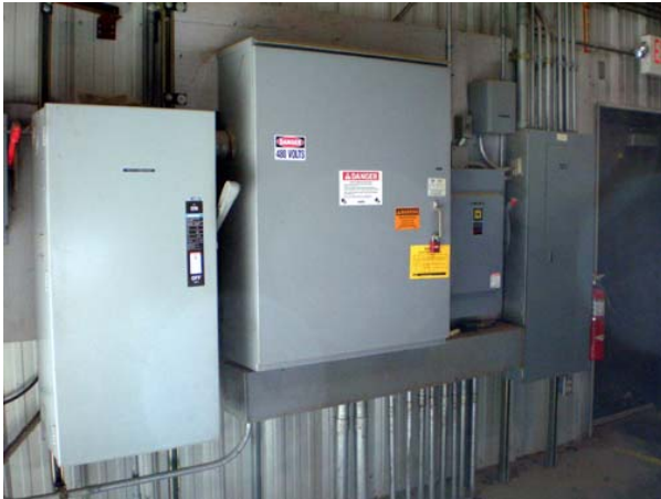
Figure 1 Electrical Subpanels (inside)
