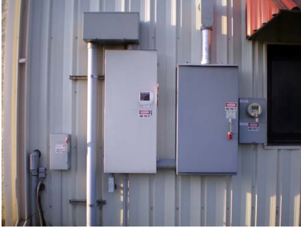
Figure 3 Electrical Service (outside)
