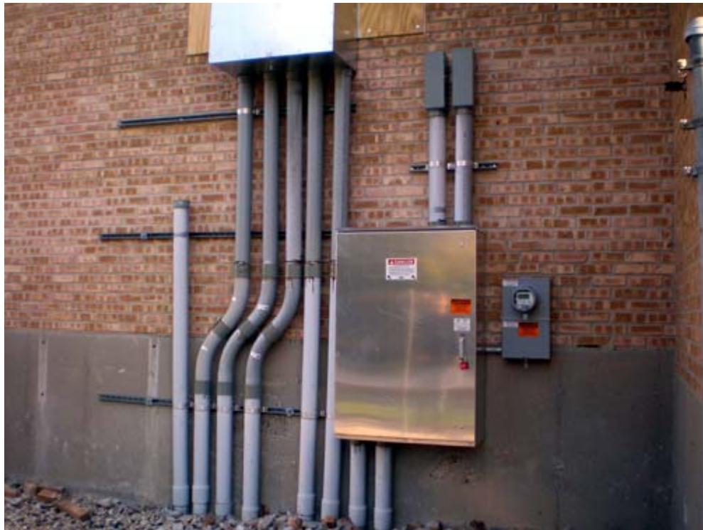
Figure 3 Electrical Service (outside)
