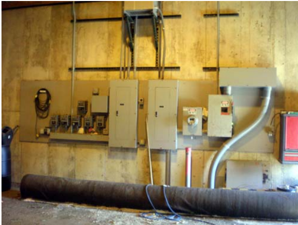
Figure 1 Electrical Subpanels (inside)
