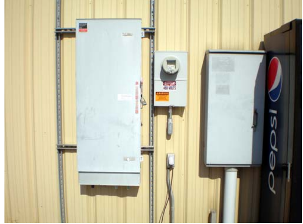
Figure 4 Electrical Service (outside)
