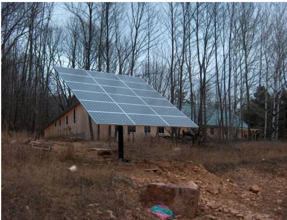
Figure 13 Example of a 3.2 kW pole mounted, fixed array that is seasonally adjustable.
