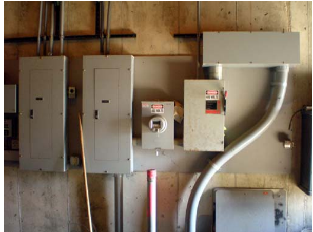
Figure 2 Electrical Subpanels (inside)
