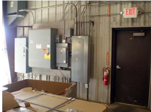
Figure 2 Electrical Subpanels (inside)
