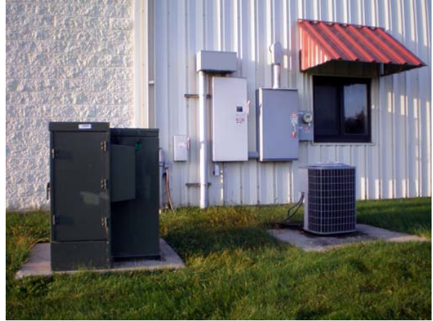
Figure 4 Electrical Service (outside)
