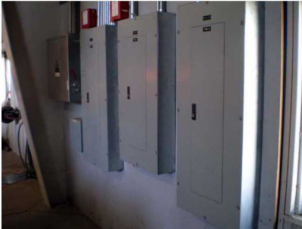
Figure 1 Electrical Subpanels (inside)
