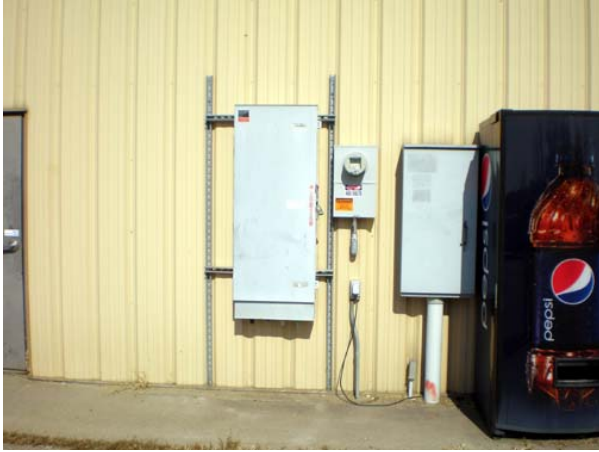
Figure 3 Electrical Service (outside)
