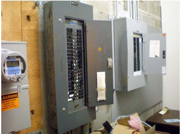
Figure 1 Electrical Subpanels (inside)
