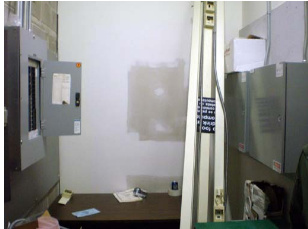
Figure 2 Electrical Subpanels (inside)
