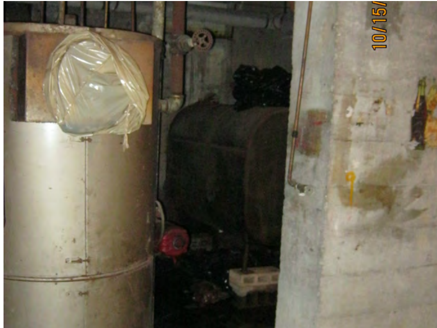
Photo 7: View of the AST observed in the basement of the 1326 Washington Avenue building
