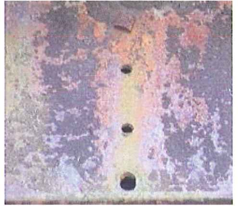
Paint on steel girder
