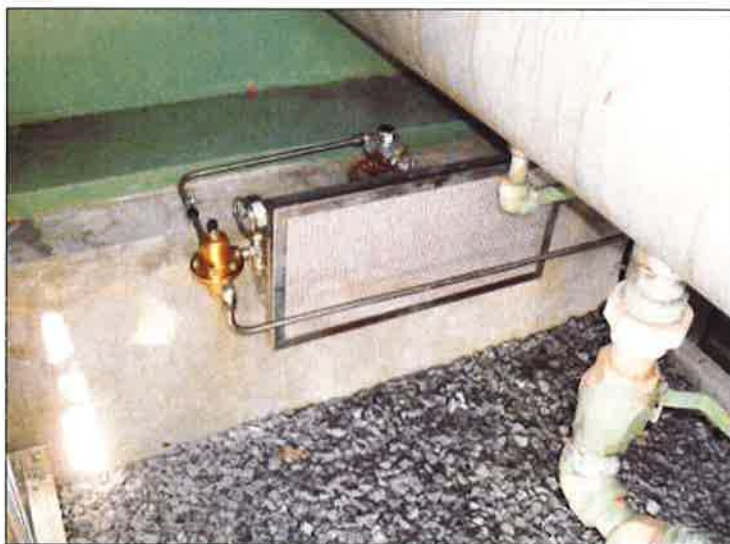
Figure 2-1: Enclosure Interior Detail
