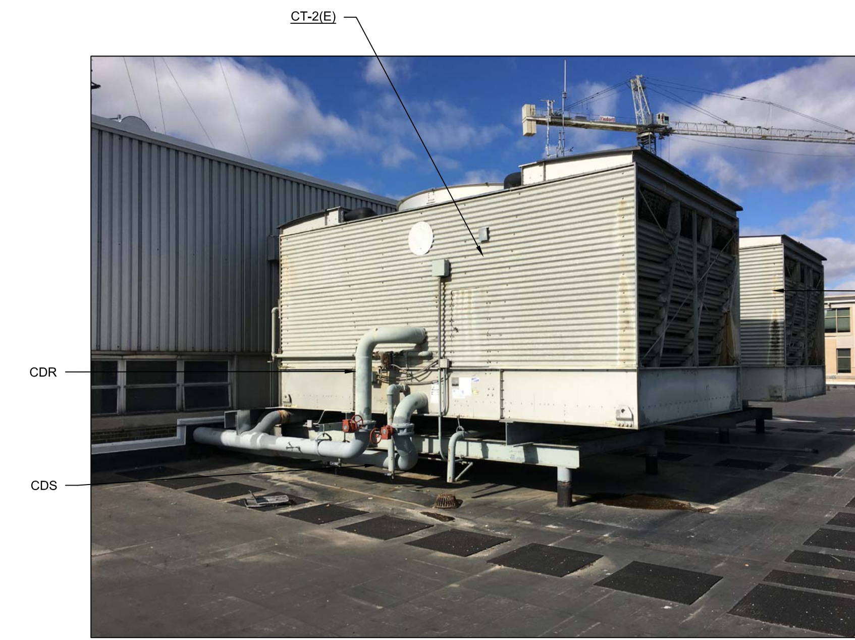
2 PHOTO - COOLING TOWER - LOOKING WEST ME101 SCALE: N.T.S.
