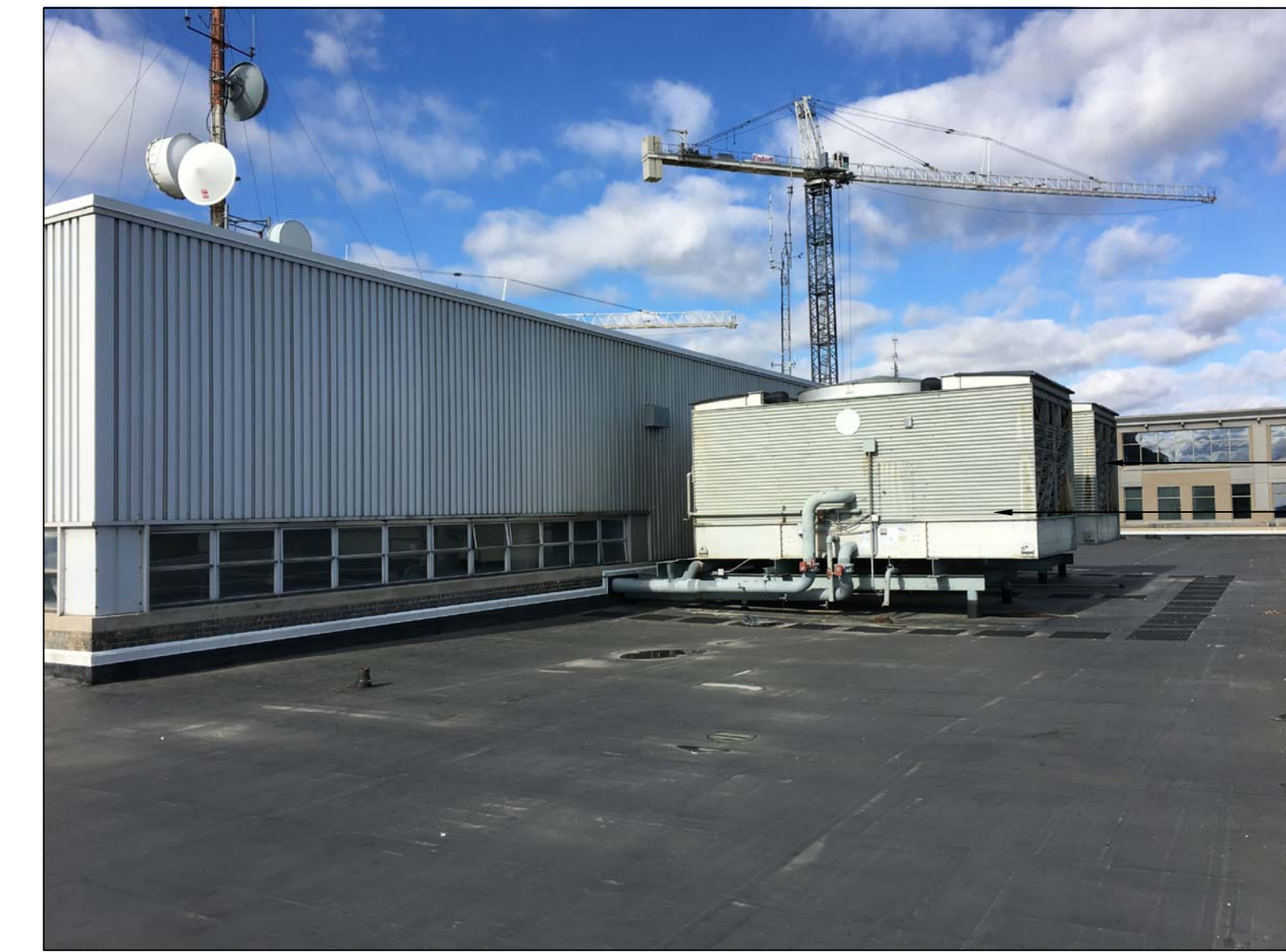
1 PHOTO - COOLING TOWER - LOOKING WEST ME101 SCALE: N.T.S.
