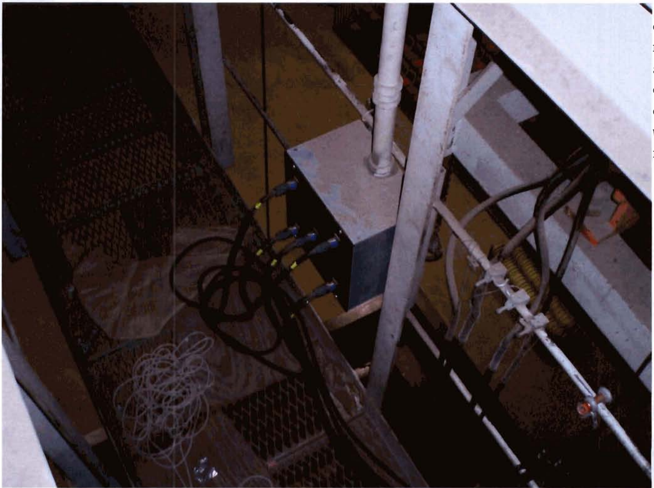
CENTER HUNG SCOREBOARD CATWALK CONTROL WIRING BOX (LEFT)
