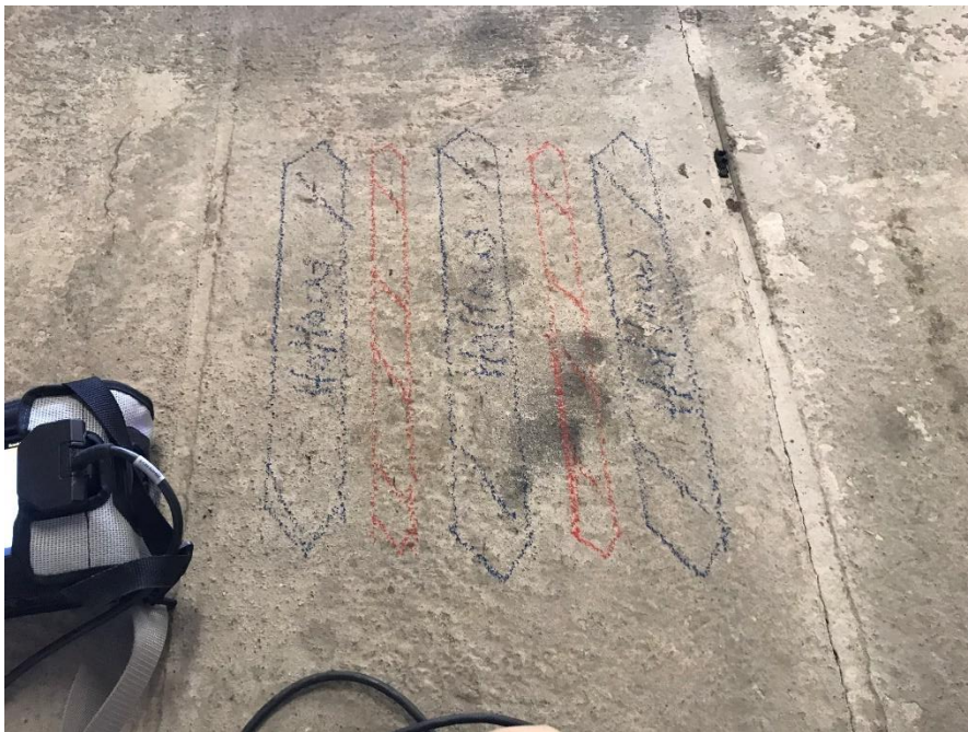
Area #10- Mezzanine Precast scan. Red represents the stressed cables and blue represents the hollow cell of the precast panel.
