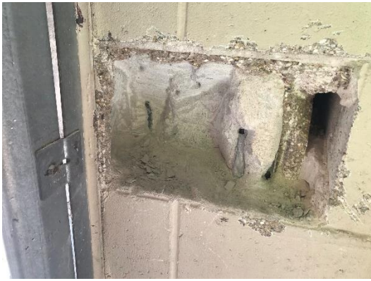
Rebar Scan #1- Rebar exposed by the customer contact.
