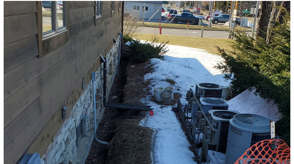
FIGURE 1.11 - EXTERIOR HVAC EQUIPMENT
