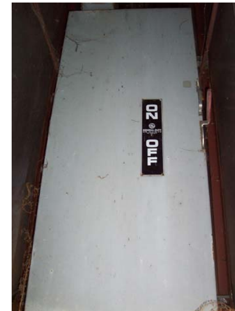
SIGN DISCONNECT SWITCH
