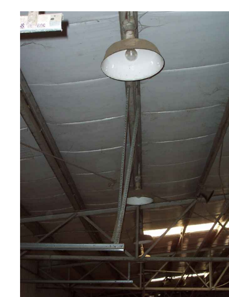
LIGHT AT OVERHEAD DOORS (BARN 9)
