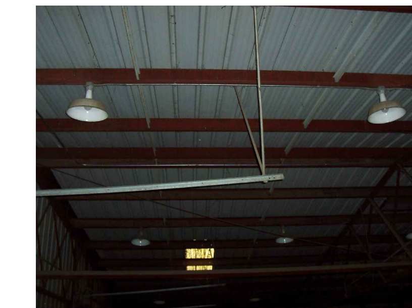
LIGHTS AT OVERHEAD DOORS (BARN 11)
