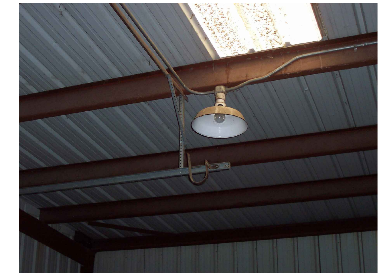
LIGHT AT OVERHEAD DOORS (BARN 3)
