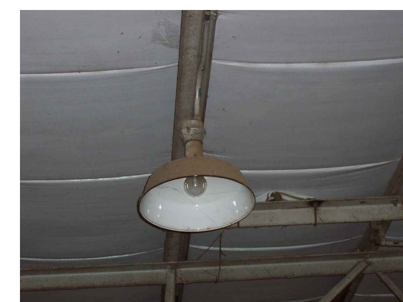
TYPICAL LIGHT (BARN 9)
