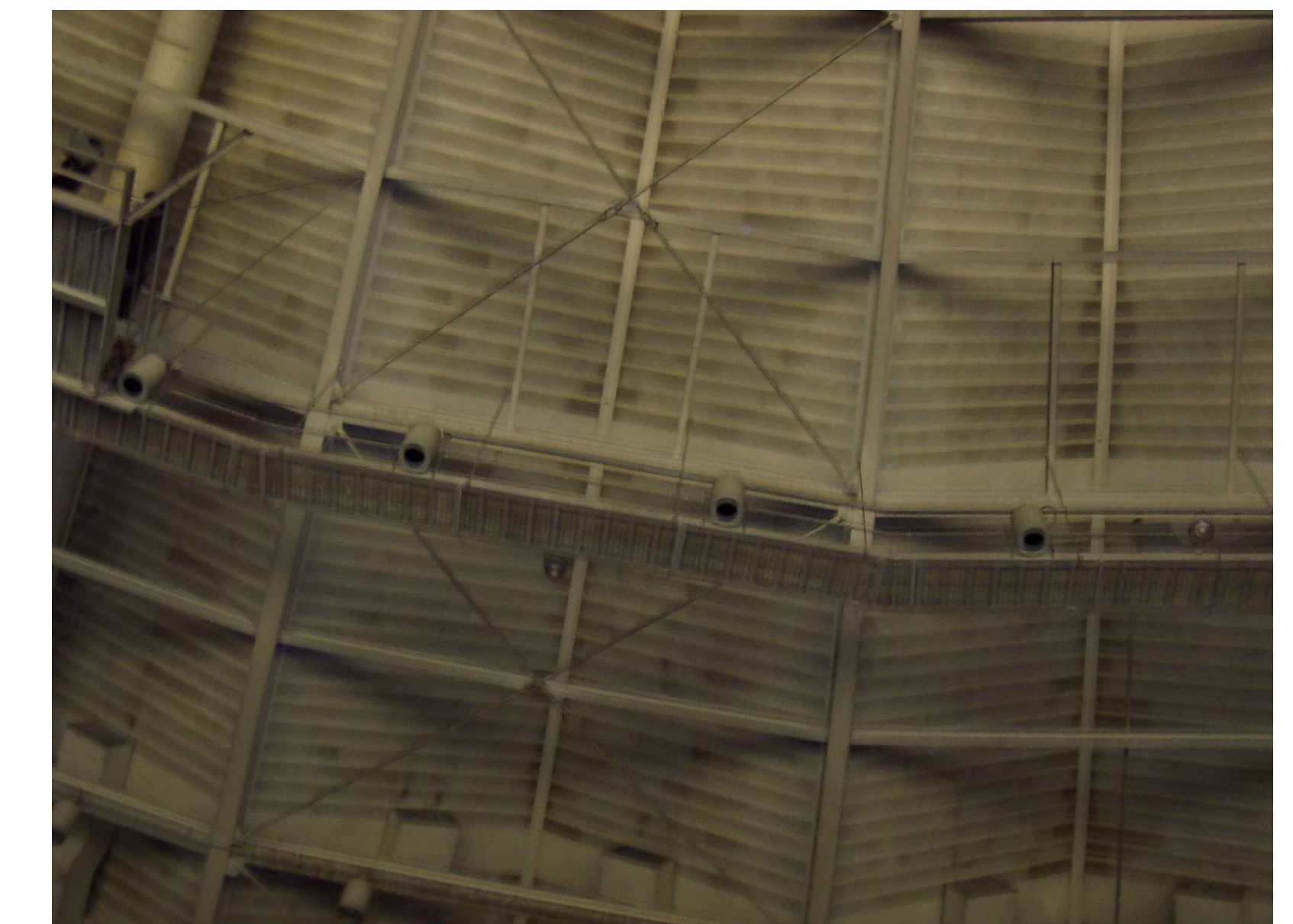
LIGHTS AT CATWALK
