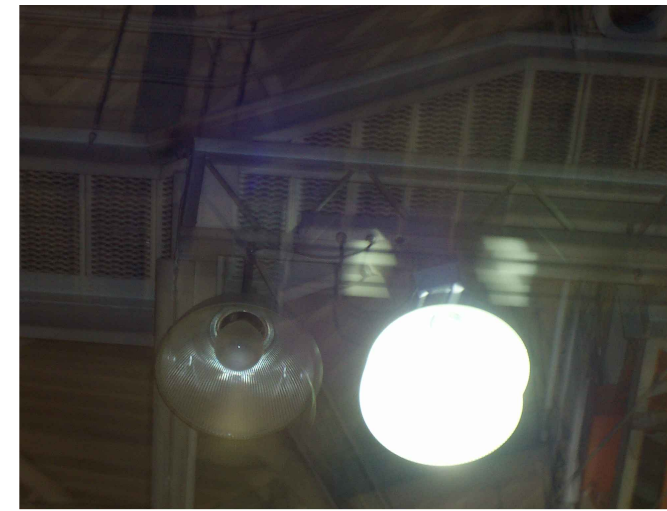
LIGHTS ON RACK OVER FLOOR
