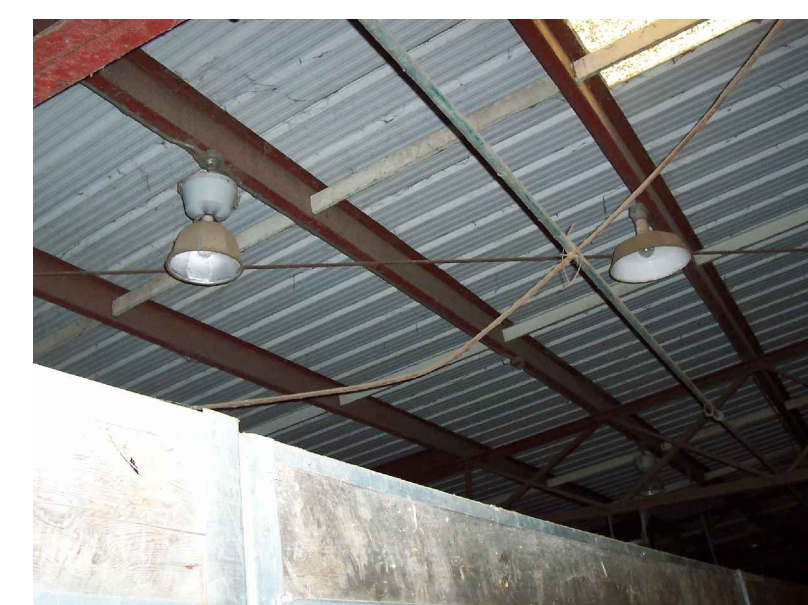
TYPICAL LIGHTS (BARN 5)
