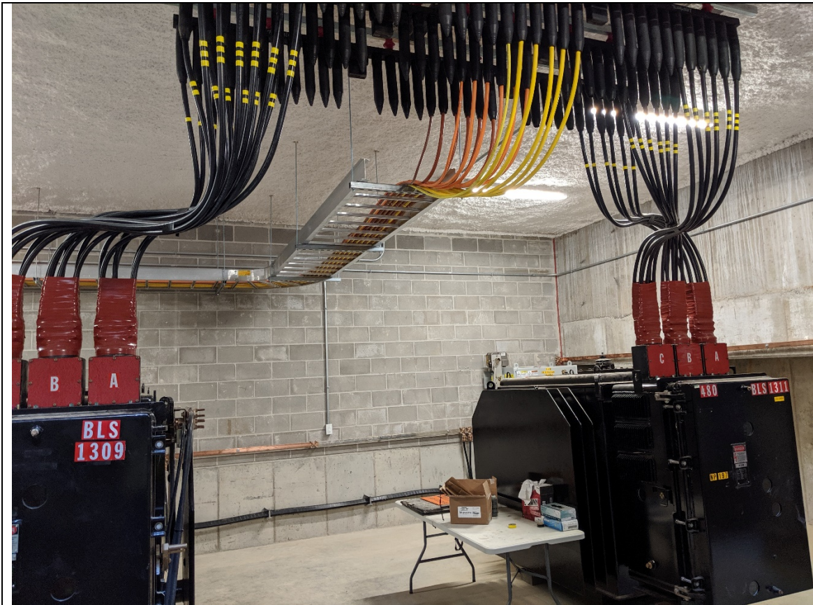
Example MG&E Vault (Not existing County Courthouse Vault) – Transformers, Collection Bus (Rockets) and Cable Tray
