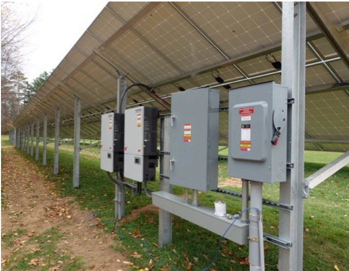
Back Side of a Ground Mounted Array. Inverters will be mounted at the array.
