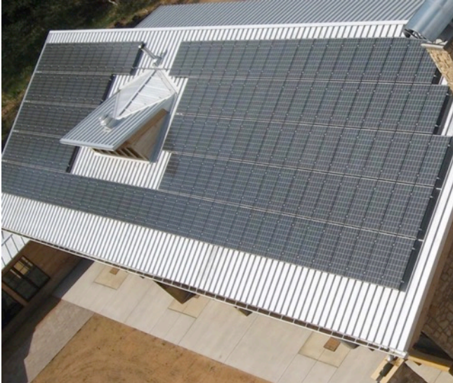
Sloping Roof Mounted
