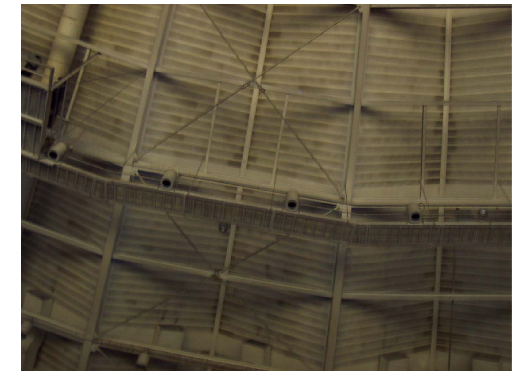
LIGHTS AT CATWALK
